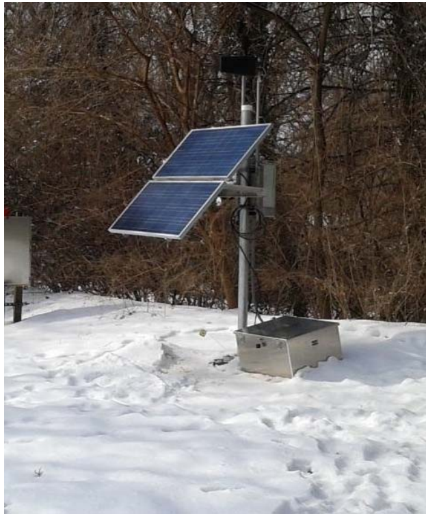
Figure 2 Solar-Powered Instrument Setup
