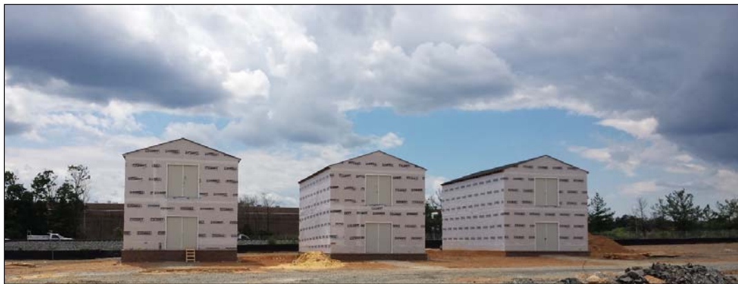
Fig. 7 – Three Completed Mockup Units – Left Building: Isolated Grade Beams & Timber Truss 1 st Floor. Center Building: Isolated Grade Beams & Hollow Core 1 st Floor, Right Building: Control Building with slab on grade foundation.
